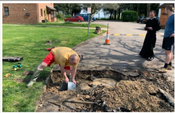
We woke up to a burst water main on Easter Monday. It seems that the old pipe, puckered and corroding in places, will need replacing very soon. 😬
